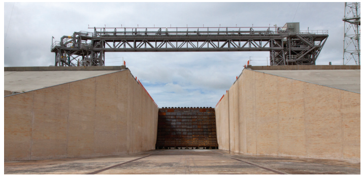
Construction is complete on the main flame deflector in the flame trench at Launch Complex 39B at NASA's Kennedy Space Center in Florida. Photo credit: NASA/Kim Shiflett
