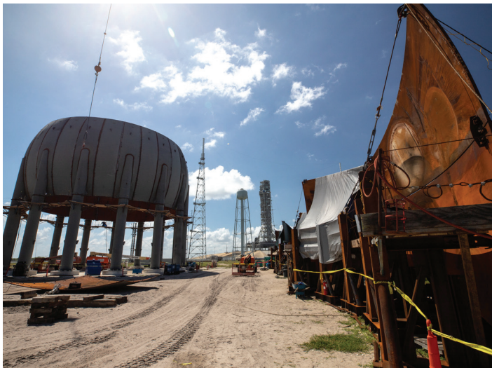
Build-up of a new liquid hydrogen (LH2) storage tank is in progress at Launch Complex 39B. The new tank will hold 1.25 million gallons of usable LH2 to support future launches, including Artemis missions to the Moon and on to Mars. Photo credit: NASA/Cory Huston
