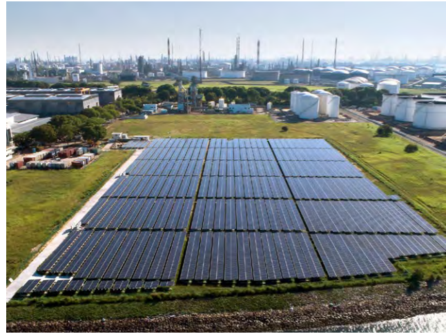
Aerial view of solar panels installed at Jurong Island
