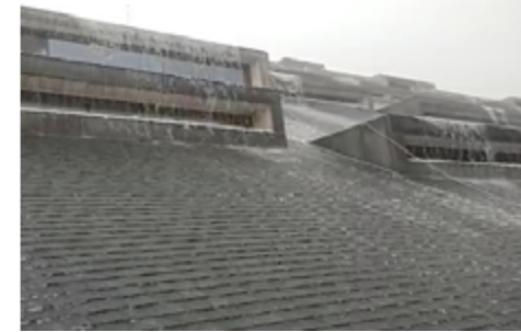
Around 18.5 lakh sq. ft. of roof area enabled with rainwater harvesting
