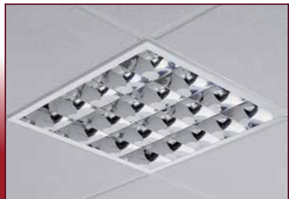
Example of converted emergency light
