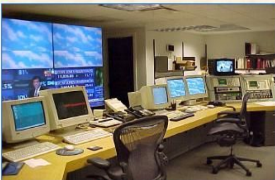
7 th Floor Comm. Room Washington, DC
