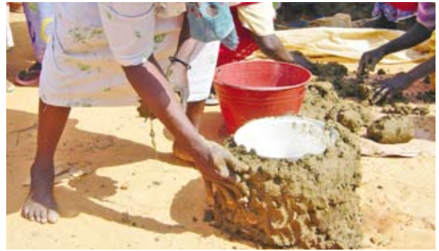
Pic 58. The pan is then placed on top of the bricks and the walls are built up until they are just under the top of the pan. Their should be a finger size gap between the pan and the wall.
