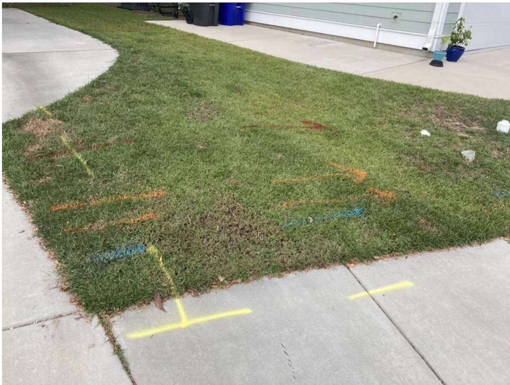
Aii Image 4: Four of five local utility markings completed on site. Fifth unmarked at time of photo.
