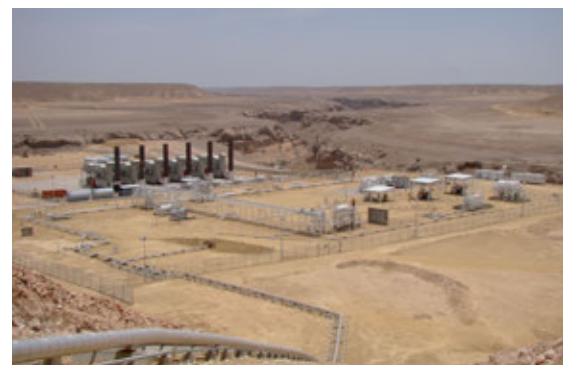
Plant in Yemen which generates electricity from associated gases that is supplied to the neighboring communities.
