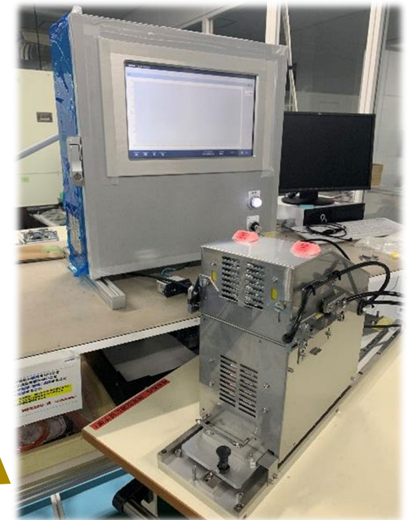
The analysis part of the X-ray analyzer being installed in the production line
