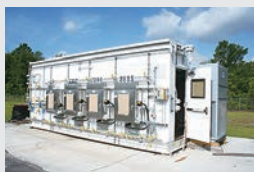
Process measurement equipment (Management of petroleum refining process)
