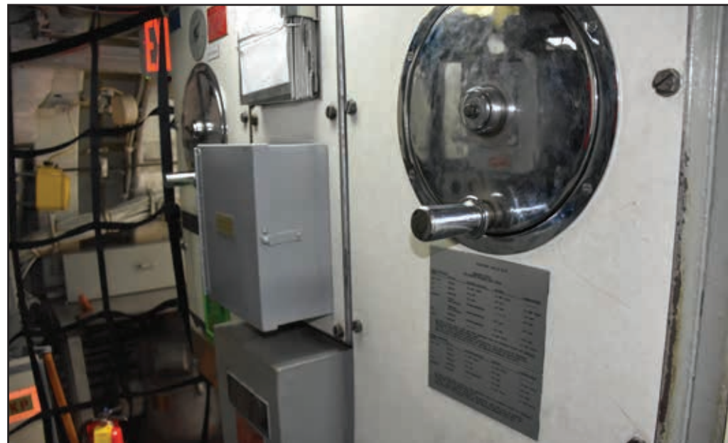
Controls for the two diesel-electric motor sets. Most engine and electrical controls are forward in the control room.
