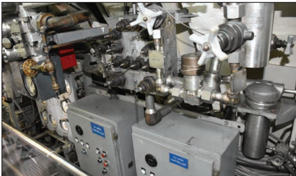
Air control systems (HPAC) stations in the engineering space.
