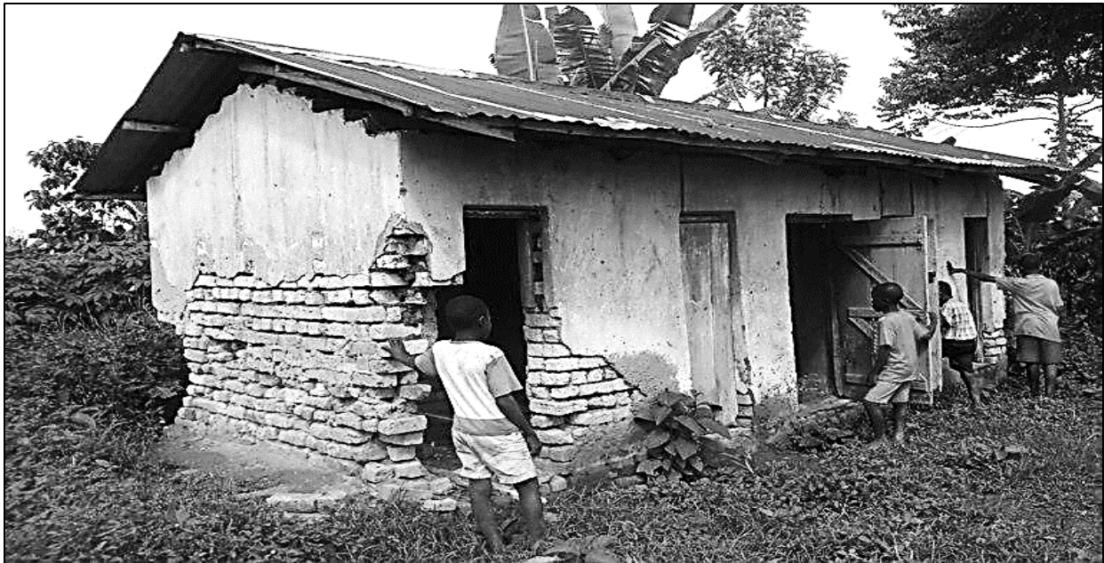
Figure 4. Universal Primary Education pupils at Katyo catholic primary school, Kalungu district in Uganda share broken bathrooms. More boys and girls in Uganda's UPE plan shy away from schooling because of poor sanitary conditions (Agaba, 2014, July 2). Retrieved from: http://www.redpepper.co.ug/challenges-in-universal-primary-education .
