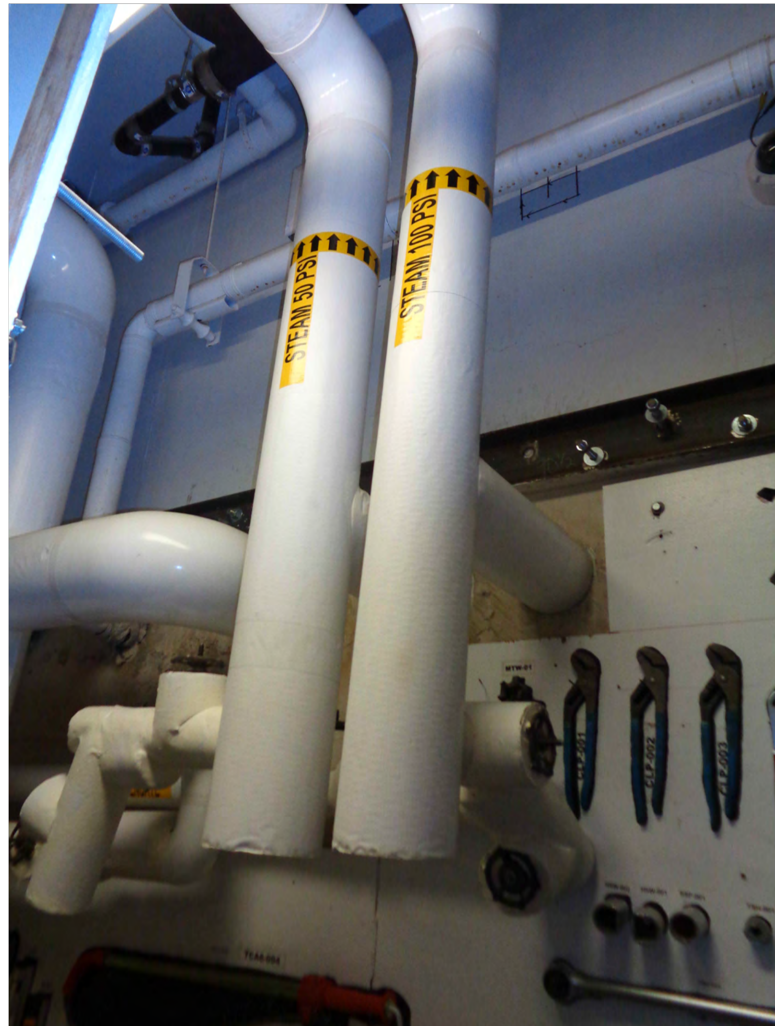
5 PIPING AT TUNNEL WALL
