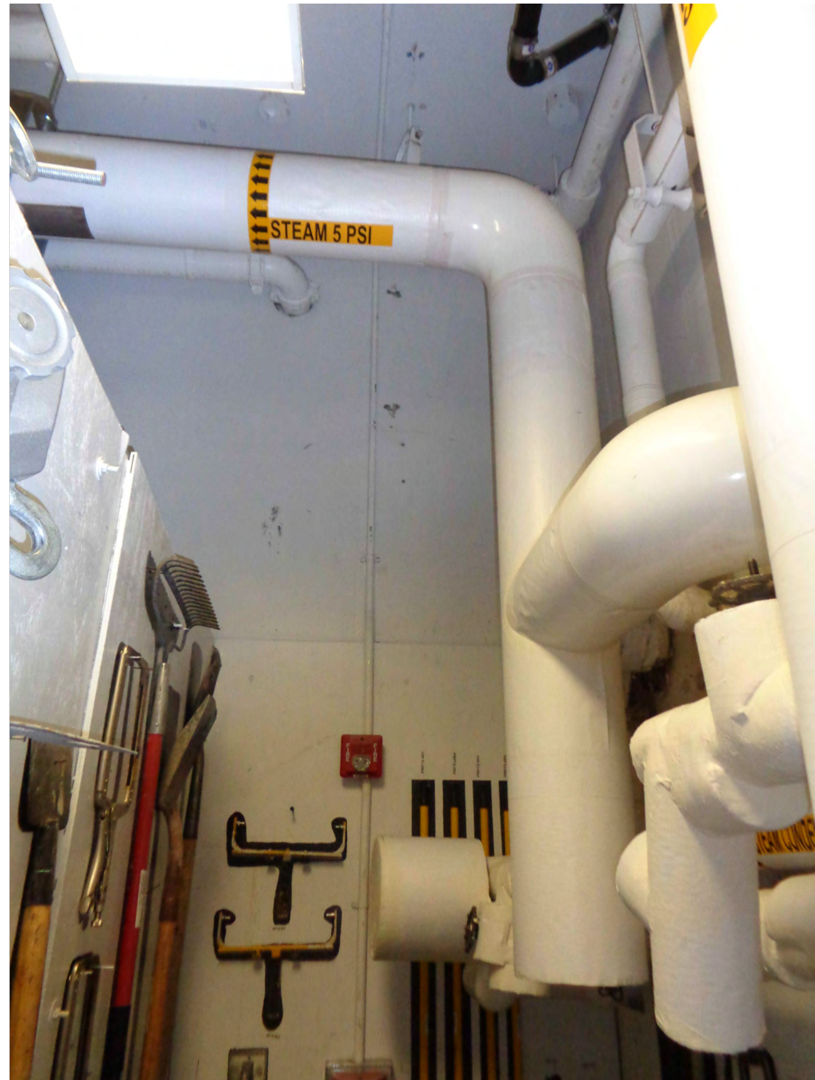
6 PIPING AT TUNNEL WALL
