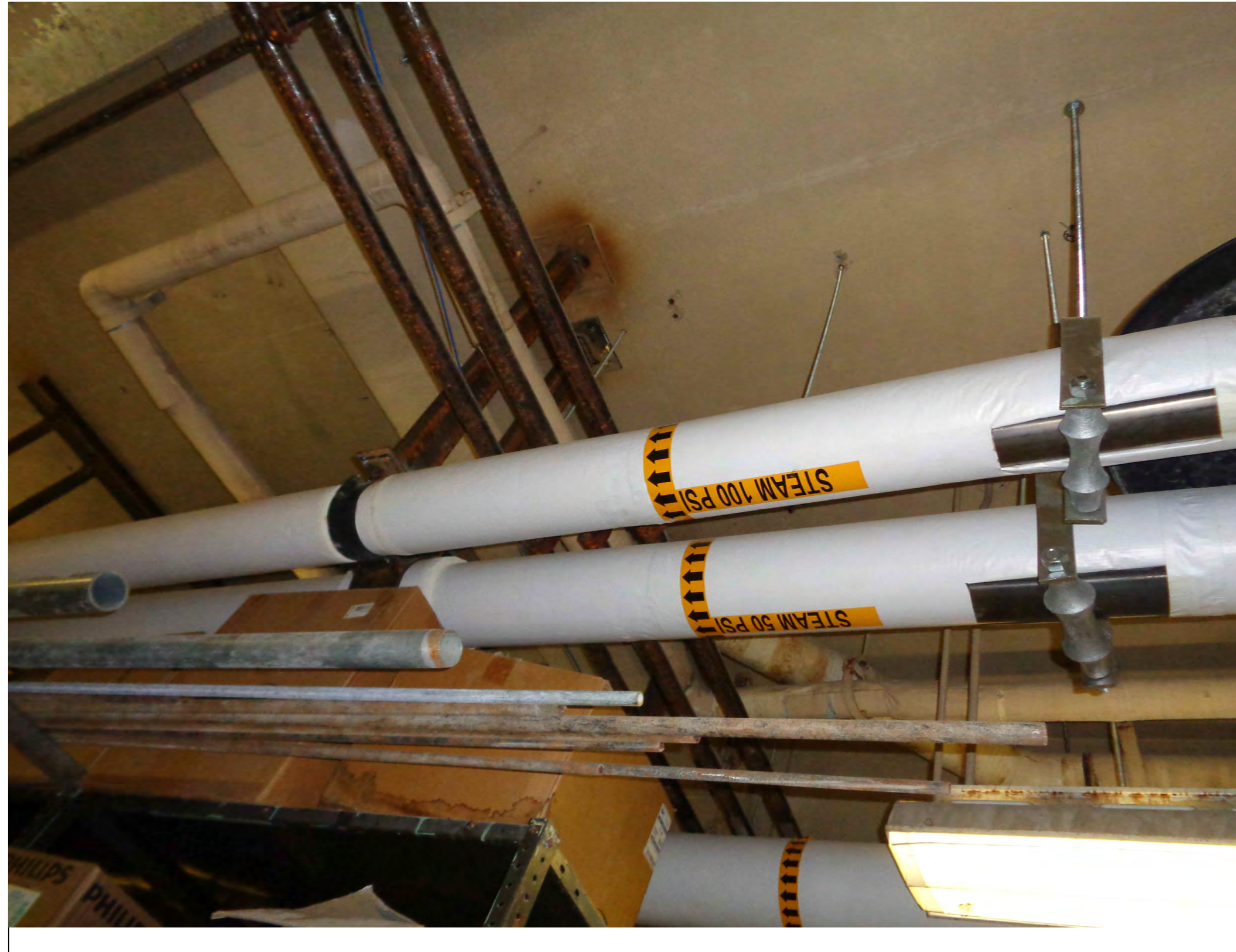
1 OVERHEAD PIPING W/ PIPE GUIDE AND PIPE HANGER
