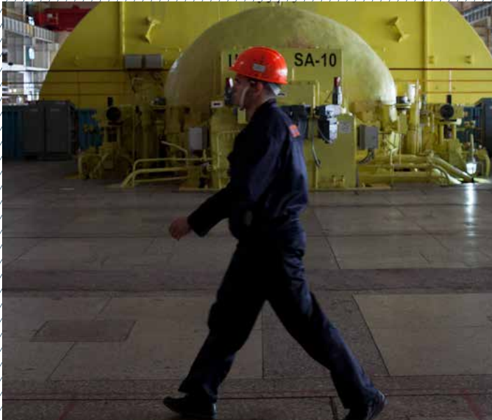
Worker at the Zaporizhska nuclear power plant in Ukraine
