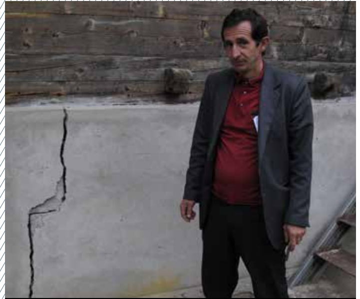
A local in Shuakhevi details the damage the construction of a nearby hydropower plant is having on the foundation of his home
